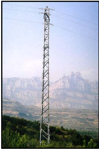
Figure I: Steel power pole that has very high risk of electrocution for the birds, placed in an area affected by forest fires. Bages (Barcelona).
